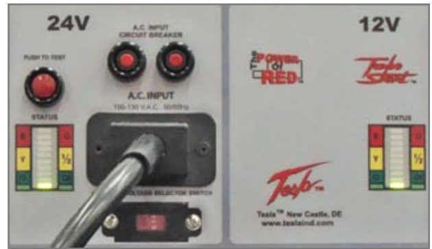
Figure 3.12.2 - AC Power Connected with LEDs Illuminated
