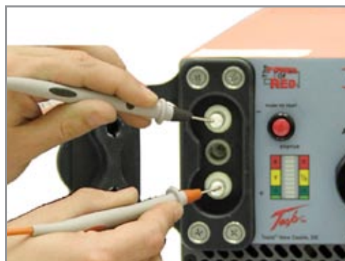
Figure 3.8.3 – Testing DC Receptacle
