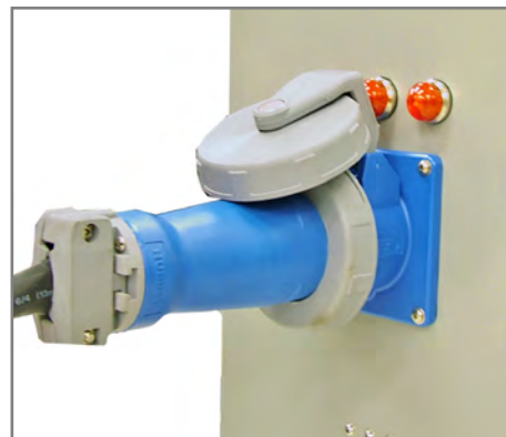
Figure 4.3.3 208 VAC cable plugged in.
