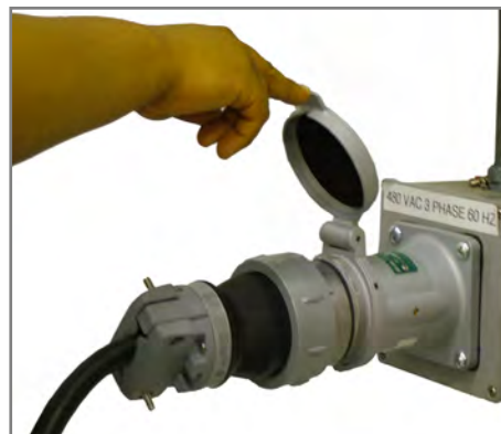
Figure 4.2.2 480 VAC cable plugged in.
